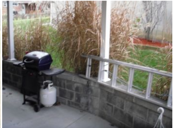
No deficiencies noted with the retaining wall in front of home or block wall along side of carport. Block wall was recently replaced.
