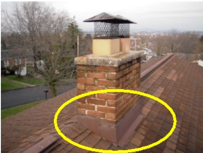
Moisture on chimney in attic indicates moisture intrusion possible through flashing around chimney exterior. Recommend sealing around flashing by a qualified roofing contractor.
