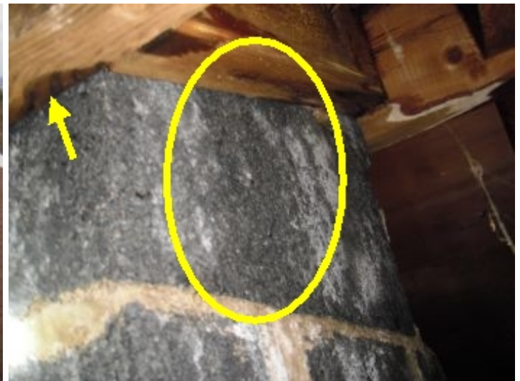
Moisture on chimney surface in attic.
