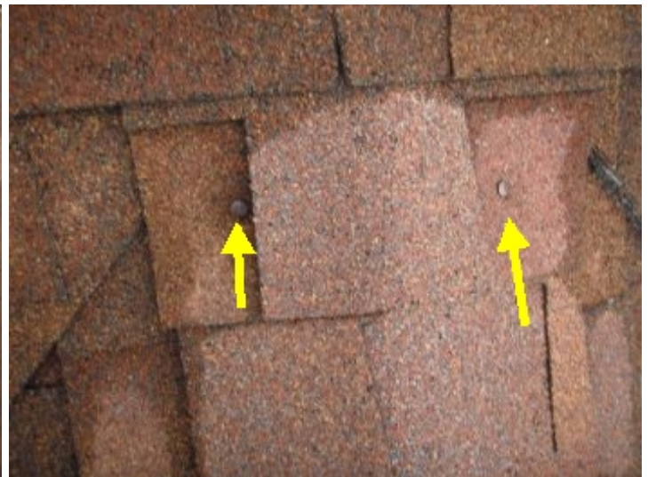
Exposed nail heads should be sealed to prevent water intrusion.
