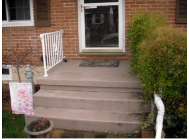
Recommend railing on front entrance steps.
