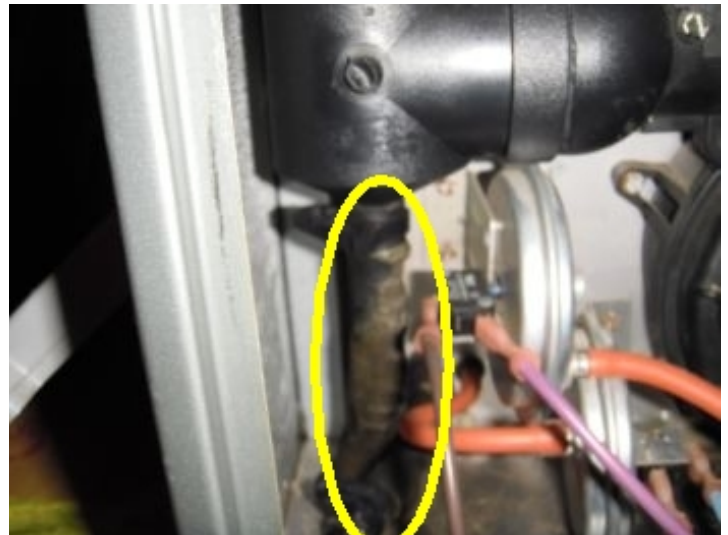
Condensate hose on furnace is leaking and must be replaced.
