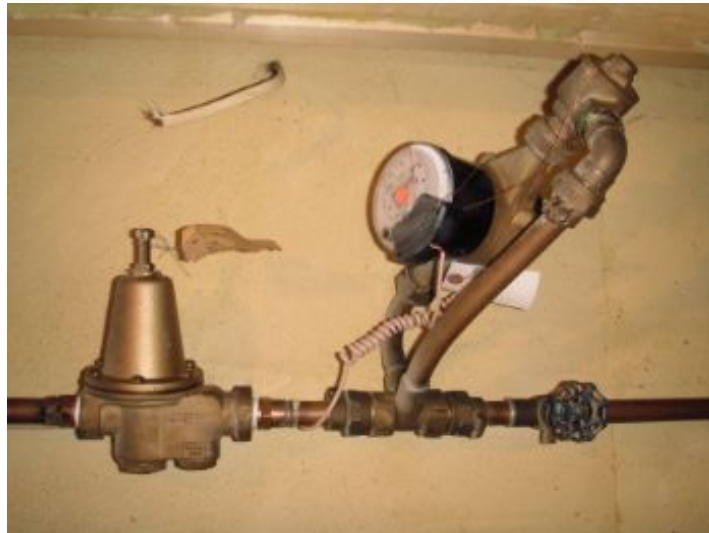
Main Water Shutoff w/ pressure reducing valve -located behind shelf in basement.
