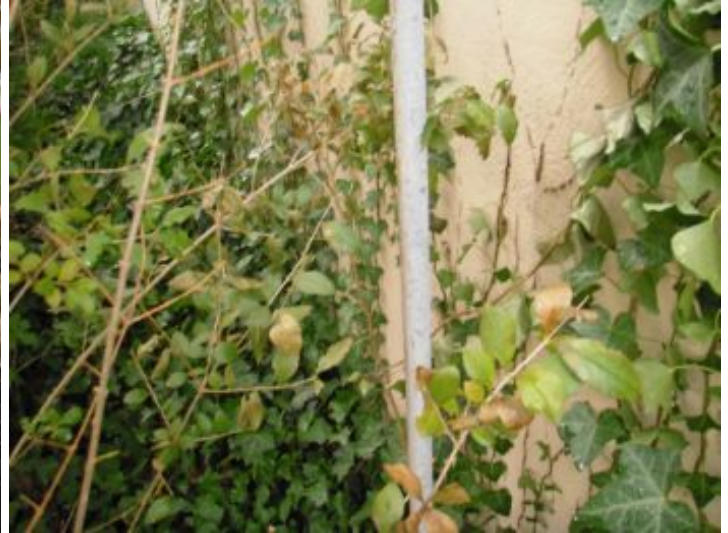
Trees and Ivy up against structure. Recommend keeping vegetation away from structure.
