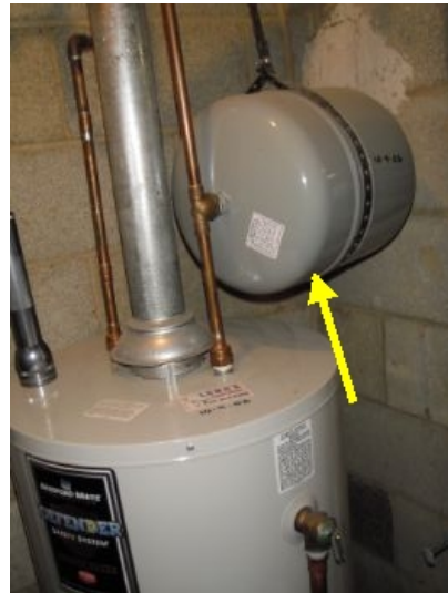
Expansion tank to protect W/H.
