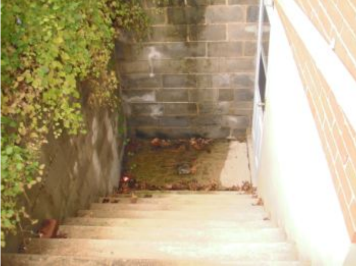
Recommend installation of a railing on steps into basement.
